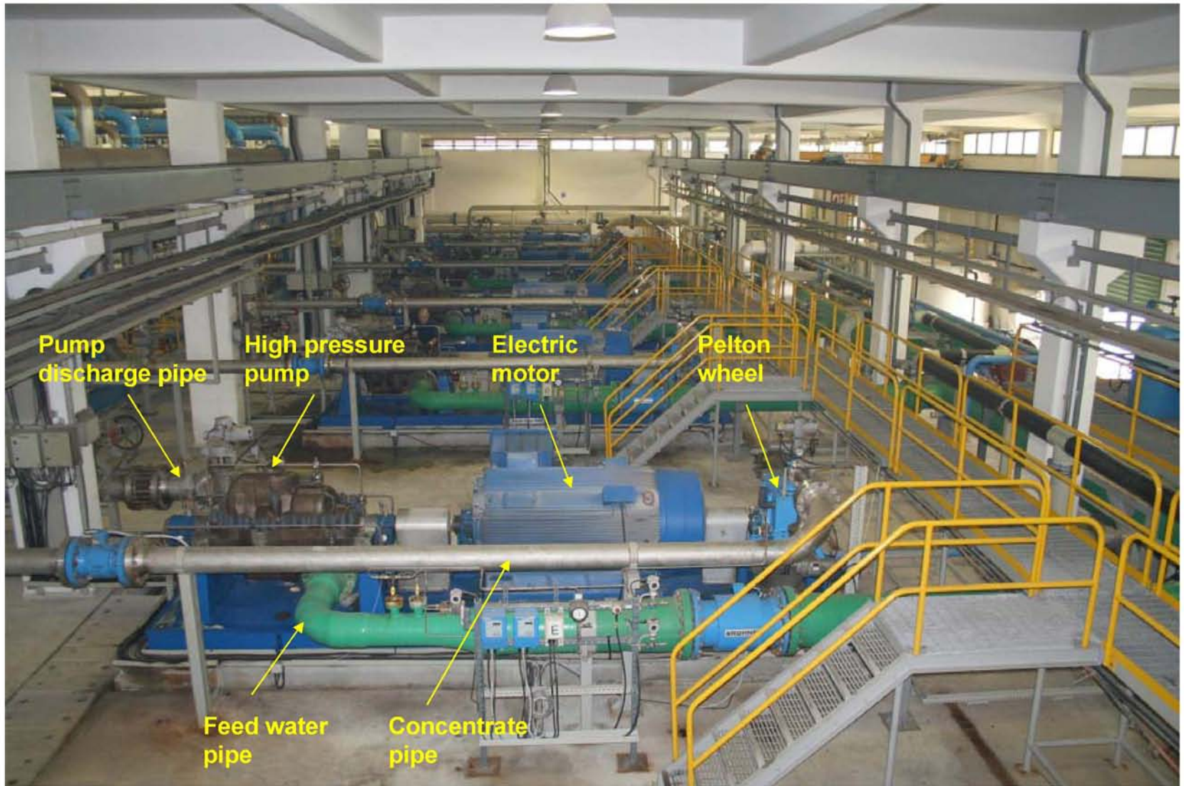
Pumping system at Larnaca plant. (Cyprus)
