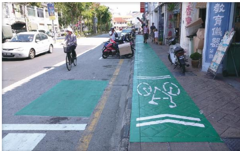
Figure 24. A bi-directional bicycle lane, painted green, was recently implemented in George Town. Photo credit: Phil Tinn, 2016
