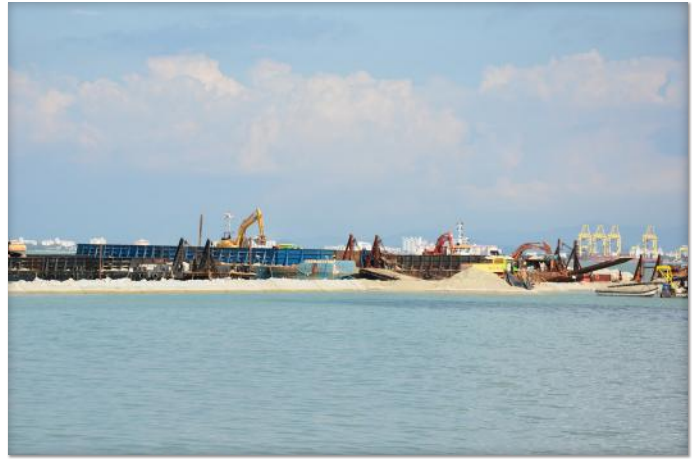
Figure 23. Coastal land reclamation has been used in Penang Island to make land available for development, such as the Seri Tanjung Pinang reclamation project in the north. Photo Credit: Sera Tolgay, 2017
