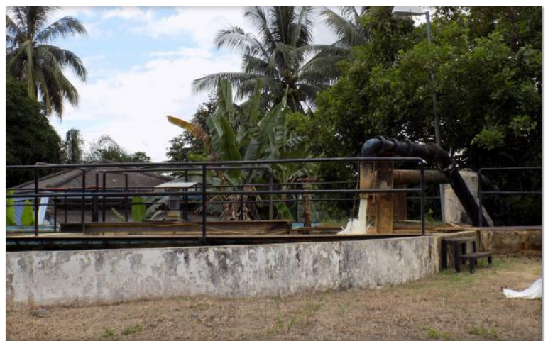
Figure 37 . Drinking water treatment plant in Raub, Pahang. Pahang transfers drinking water to Selangor. Photo credit: Kara Runsten, 2017.
